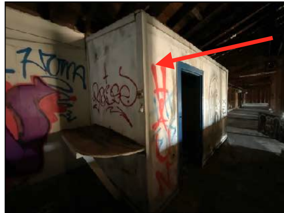
Interior, Building 2082 - Drywall/Sound Board/Fiber Board Coated With Lead-Based Paint
