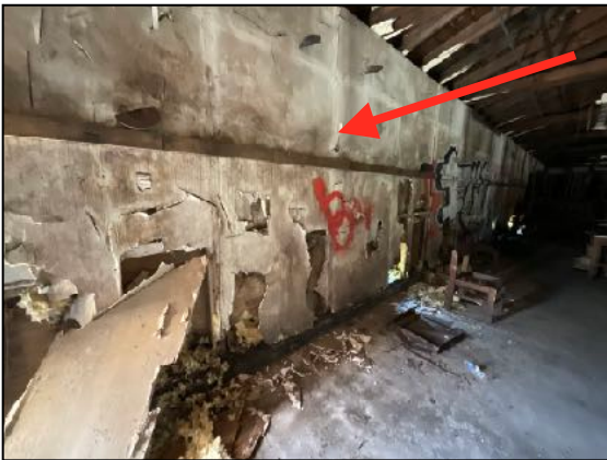
Interior, Building 2080 - Drywall Wall Coated With Lead-Based Paint
