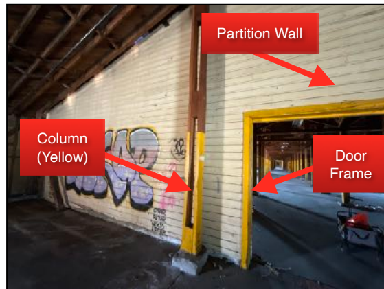
Interior, Building 2083 - Partition Wall, Column, & Door Frame Coated With Lead-Based Paint
