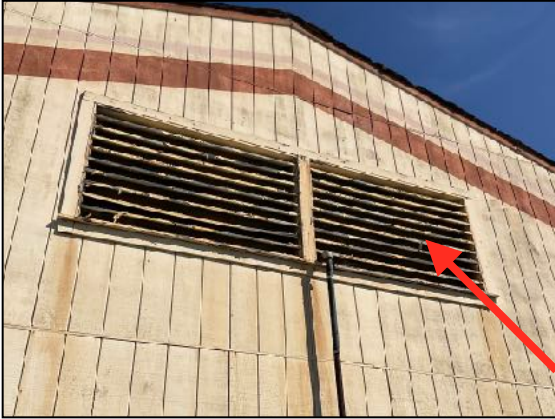
Exterior - South Louver Coated With Lead-Based Paint
