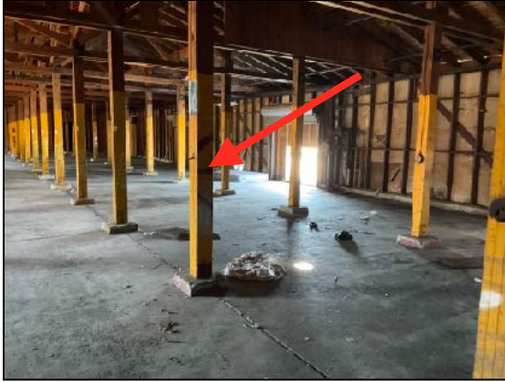
Interior, Building 2083 - Columns (Yellow) Coated With Lead-Based Paint
