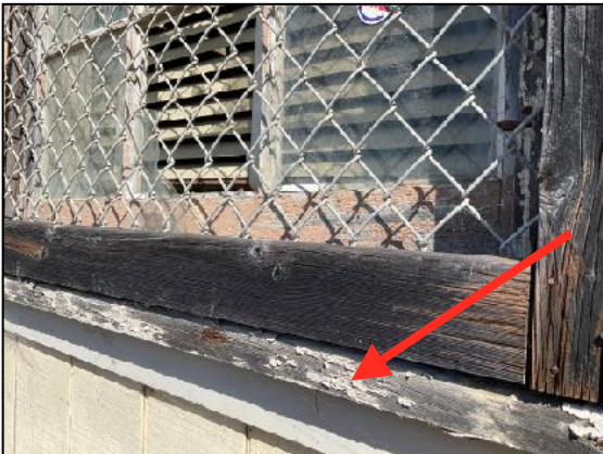
Exterior - Defective LBP On South Windows
