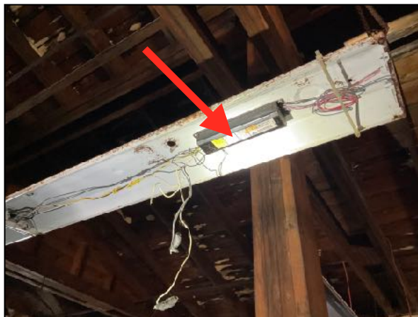
Florescent Light Fixture Ballast
