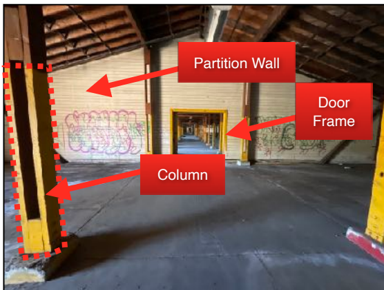
Interior, Building 2082 - Partition Wall, Column, & Door Frame Coated With Lead-Based Paint
