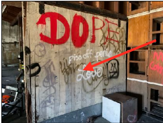
Interior, Building 2081 - Partition Wall Coated With Lead-Based Paint
