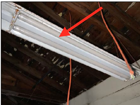
Florescent Tube Light Fixture
