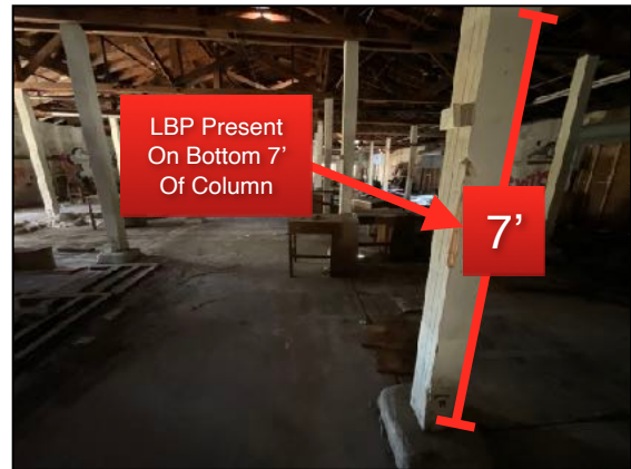
Interior, Building 2080 - Column Coated With Lead-Based Paint (LBP Present On Bottom 7')
