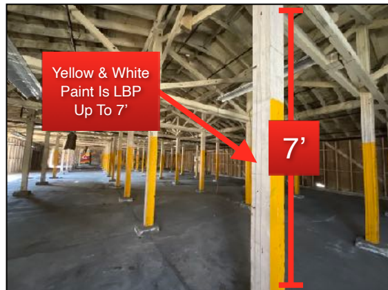
Interior, Building 2084 - Columns Coated With Lead-Based Paint (LBP Present On Bottom 7\')
