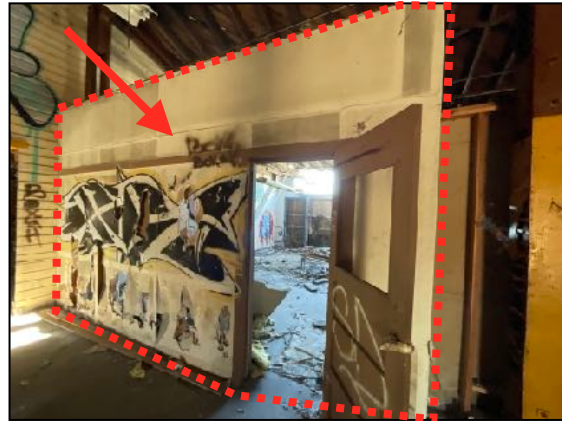
Interior, Building 2084 - Drywall/Sound Board/Fiber Board Coated With Lead-Based Paint
