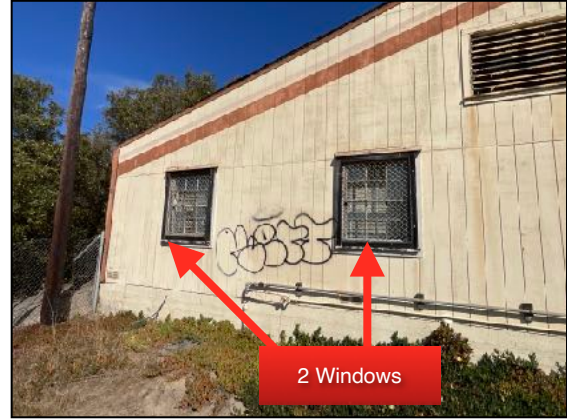
Exterior - South Window Components Coated With Lead-Based Paint
