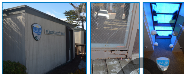
City facilities were built over 40 years ago for temporary use. Structures are decaying and plastic tarps are used to prevent roof leaks.
