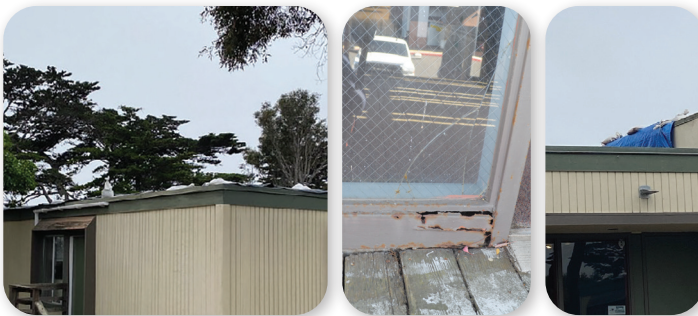
City facilities were built over 40 years ago for temporary use. Structures are decaying and plastic tarps are used to prevent roof leaks.
